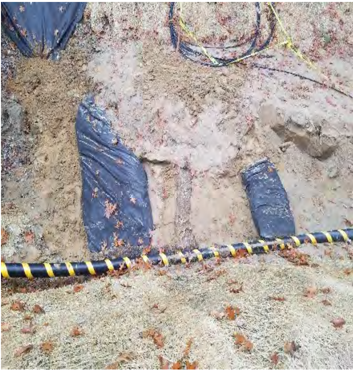
Fig 28: Crew removed sediment build up from check dam in trench at Gundalow Landing/east side of the Bay. Viewing south. (10-29-19).
