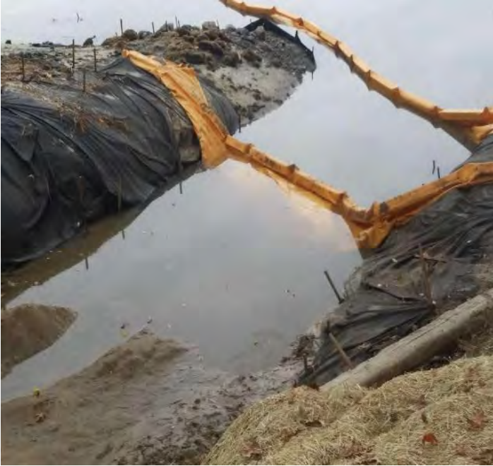
Fig 5: Two rows of silt curtain installed at Gundalow landing/east side of the Bay. Viewing west. (10-25-19).
