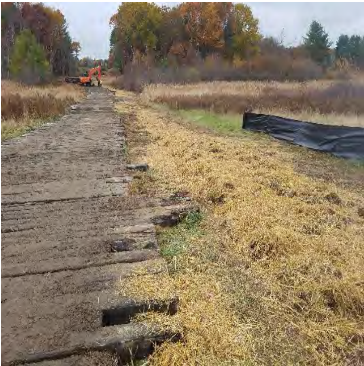
Fig 23: Crew added more straw cover over restored trench areas at Frink farm. Viewing east (10-29-19).
