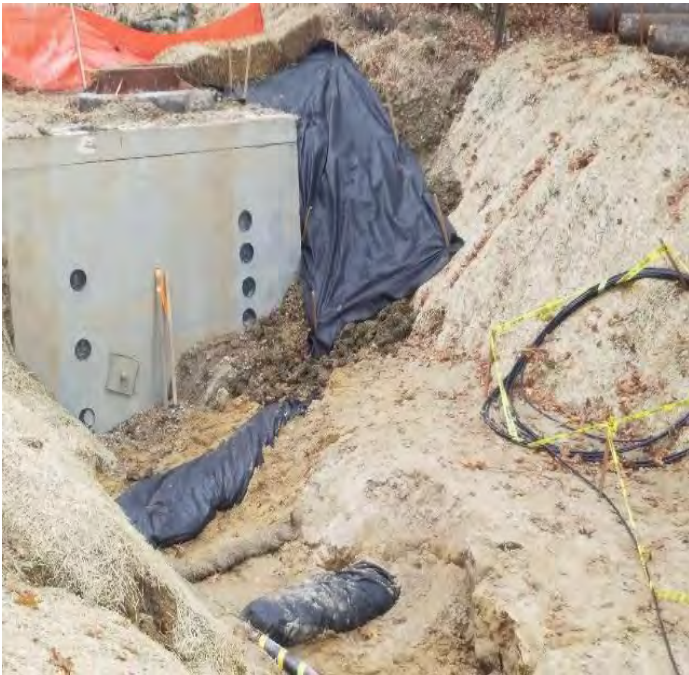
Fig 3: Trench faces in trench at Gundalow landing/east side of the Bay have been covered and secured. Viewing southeast. (10-25-19).
