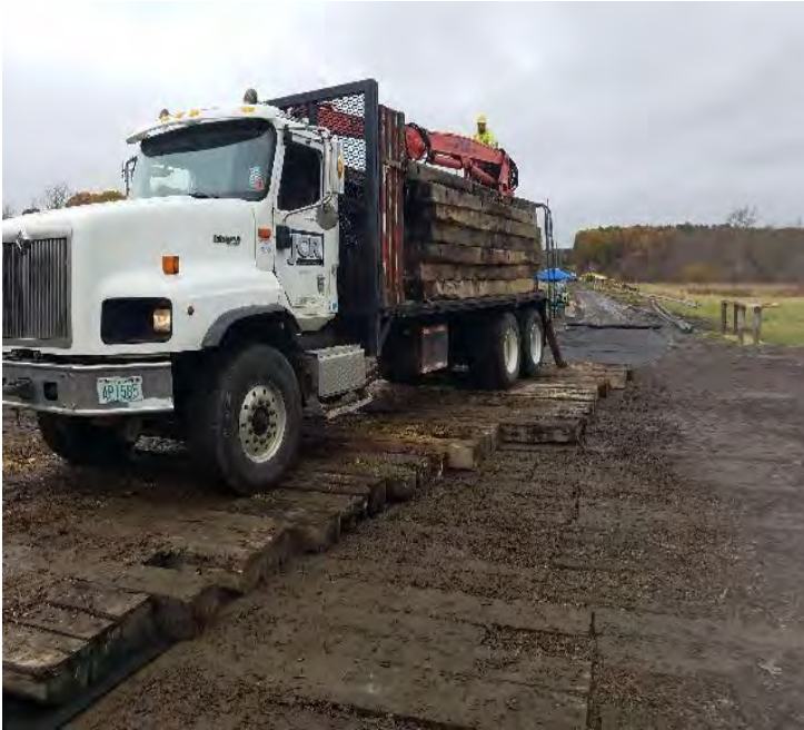
Fig 21: Crew installing second row of timber mats on access road at Frink viewing east. (10-29-19).
