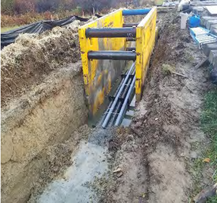
Fig 19: Groundwater in trench at Frink farm. Viewing west. (10-29-19).
