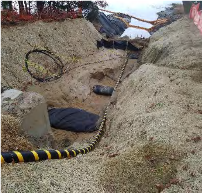
Fig 1: Berms installed in trench at Gundalow landing/east side of the Bay. Viewing west. (10-25-19).
