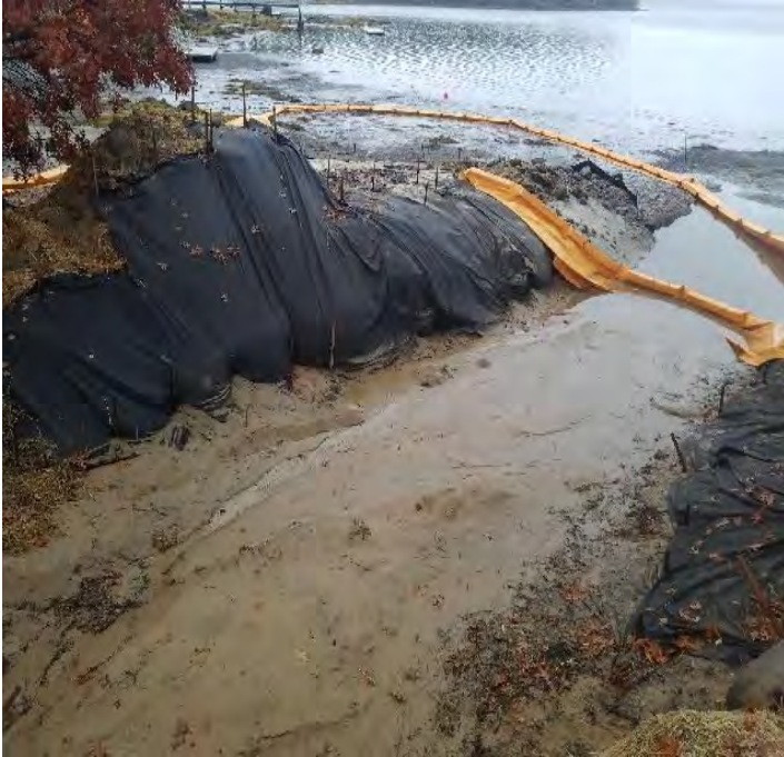
Fig 9: Trench in intertidal zone at Gundalow landing/east side of the Bay. Viewing west. (10-28-19).
