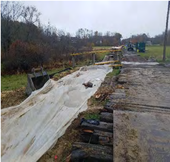
Fig 11: Exposed soils covered at Frink farm. Viewing west. (10-28-19).
