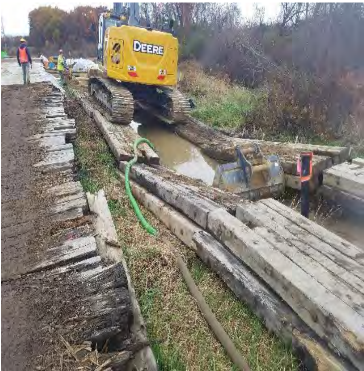
Fig 30: Pumping water out of trench in NW18 at Frink farm. Viewing east. (10-30-19).
