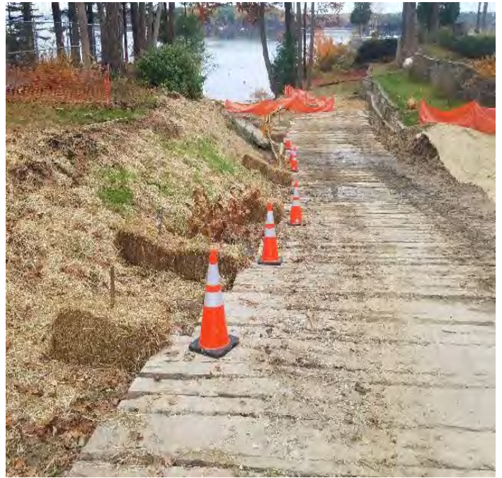
Fig 4: Straw bales installed in swale next to access to vault and trench at Gundalow landing/east side of the Bay. Viewing west. (10-25-19).
