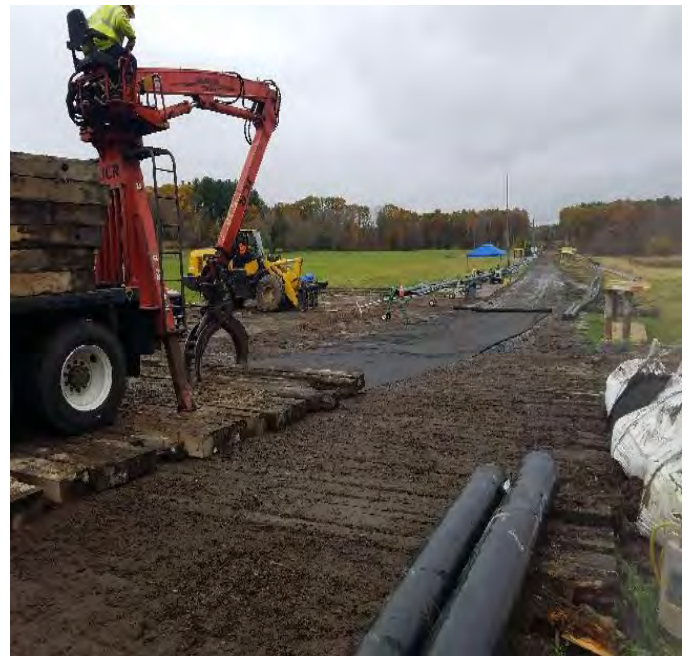
Fig 22: Crew installing second row of timber mats on access road at Frink farm. (10-29-19).
