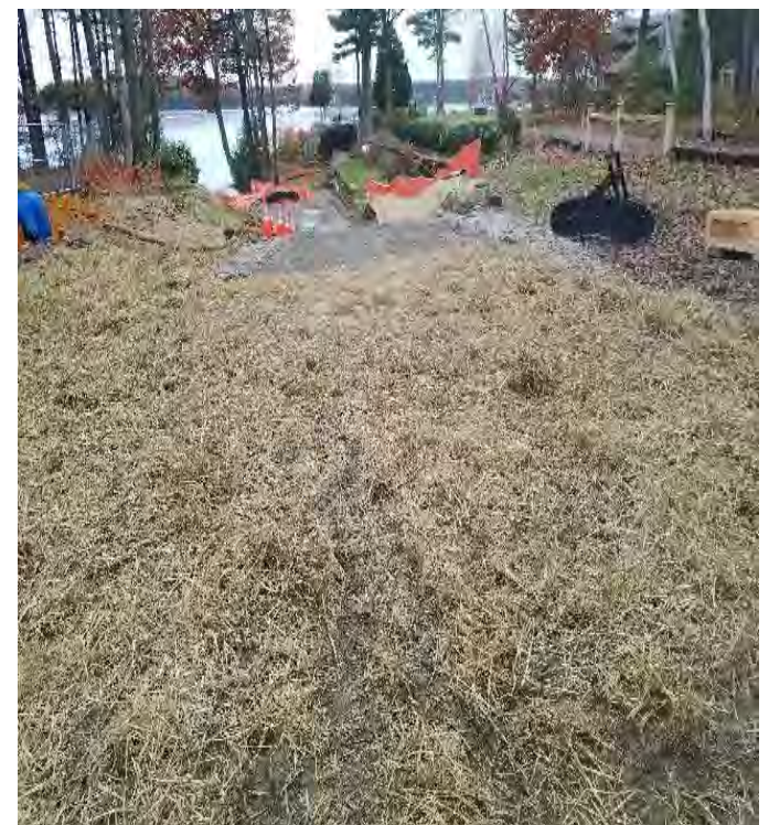
Fig 27: Access down to vault and trench at Gundalow landing/east side of the Bay. Viewing west. (10-29-19).
