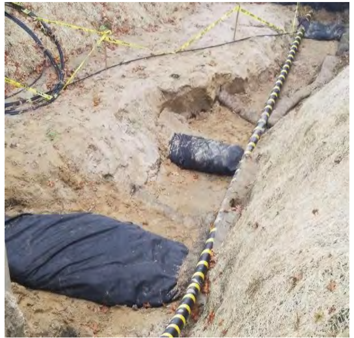
Fig 2: Berms installed in trench at Gundalow landing/east side of the Bay. Viewing west. (10-25-19).
